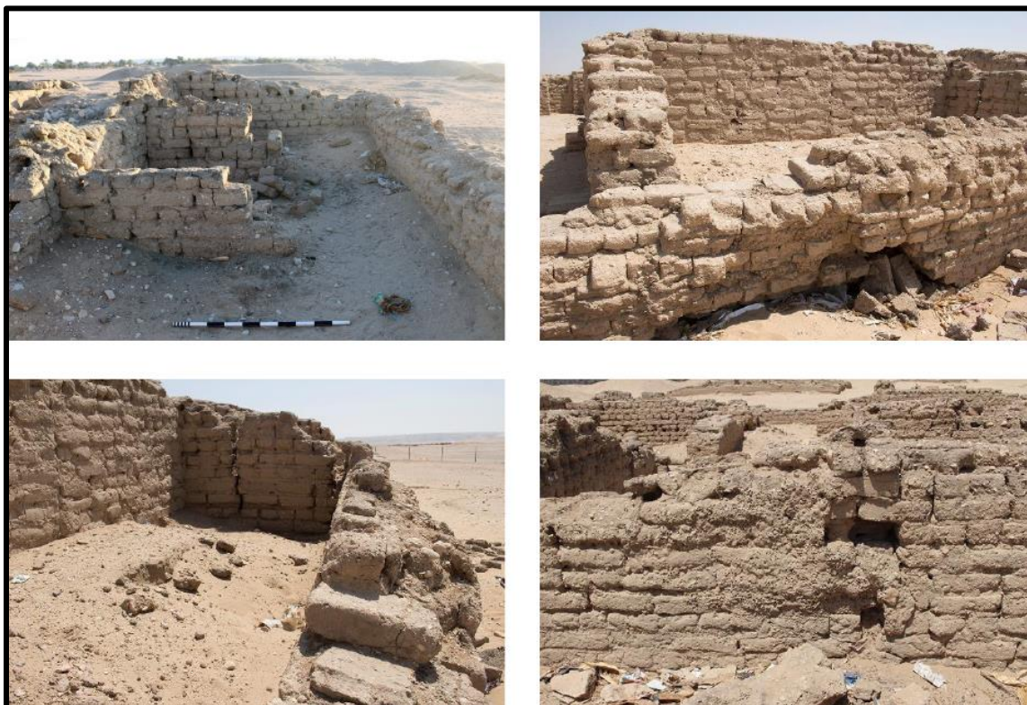
Figure 3: Crumbling, cracking and collapsing mudbrick is widespread in the exposed houses. Image courtesy of the Amarna Project.
